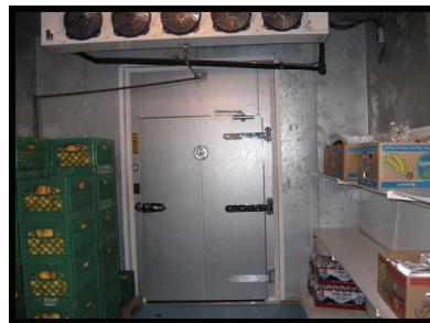
Interior View of Walk in Freezer
