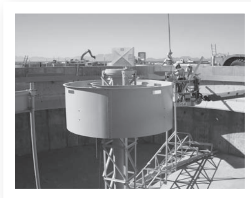
Avra Valley Clarifiers
