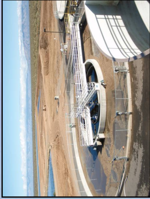
Corona de Tucson WRF - Closed Loop Reactor
